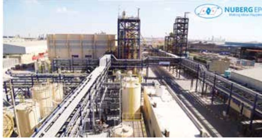
▲ Chlor Alkali Plant, Abu Dhabi.
